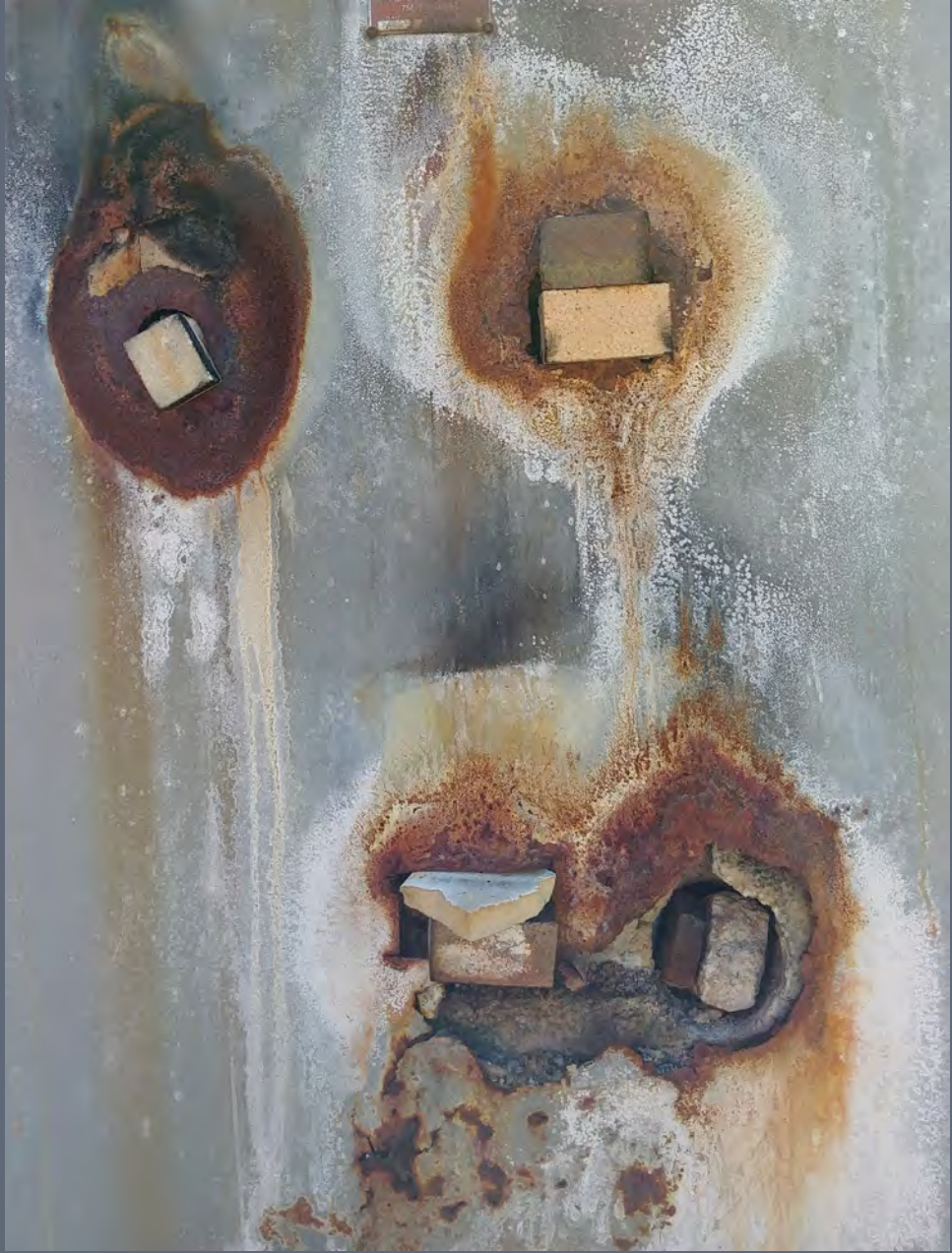
Rust, Scottsdale, Arizona
